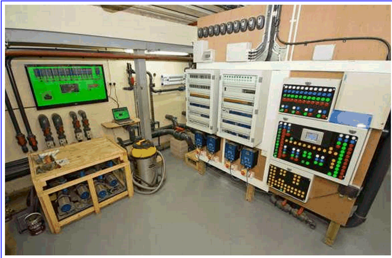
The Control Room
