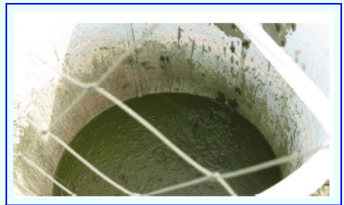
Solids Retaining Tank
